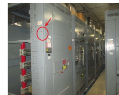
电器柜 Electric Box
